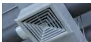
Ventilation duct monitoring
